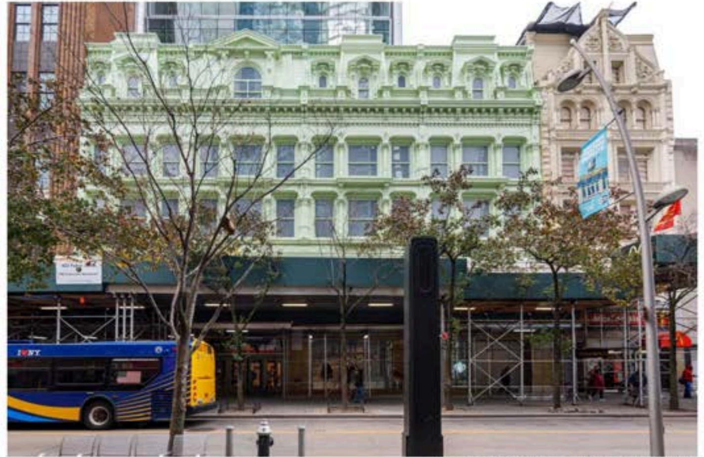
Restoration of historic cast iron facade at the base of the project
